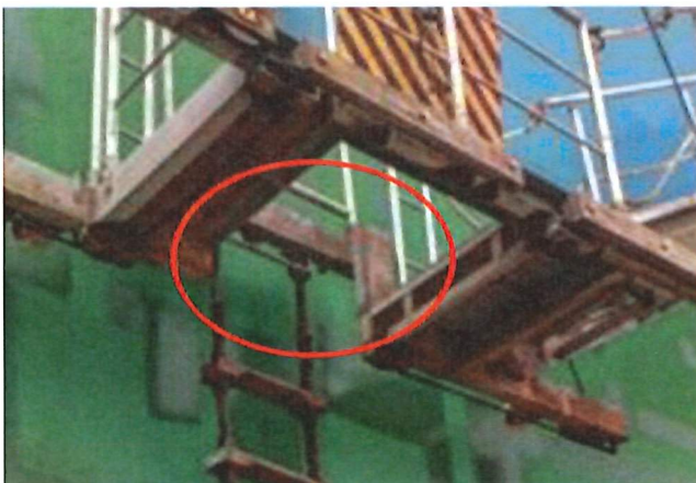
Figure 1: Pilot ladder/trapdoor showing the non-compliant horizontal cross-member.
